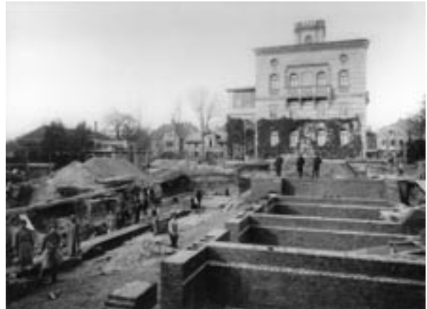
Work on the foundations of the New Castle. In the background the Old Castle, designed and built from 1844-1848 by Friedrich Bürklein, King Max II's architect.
